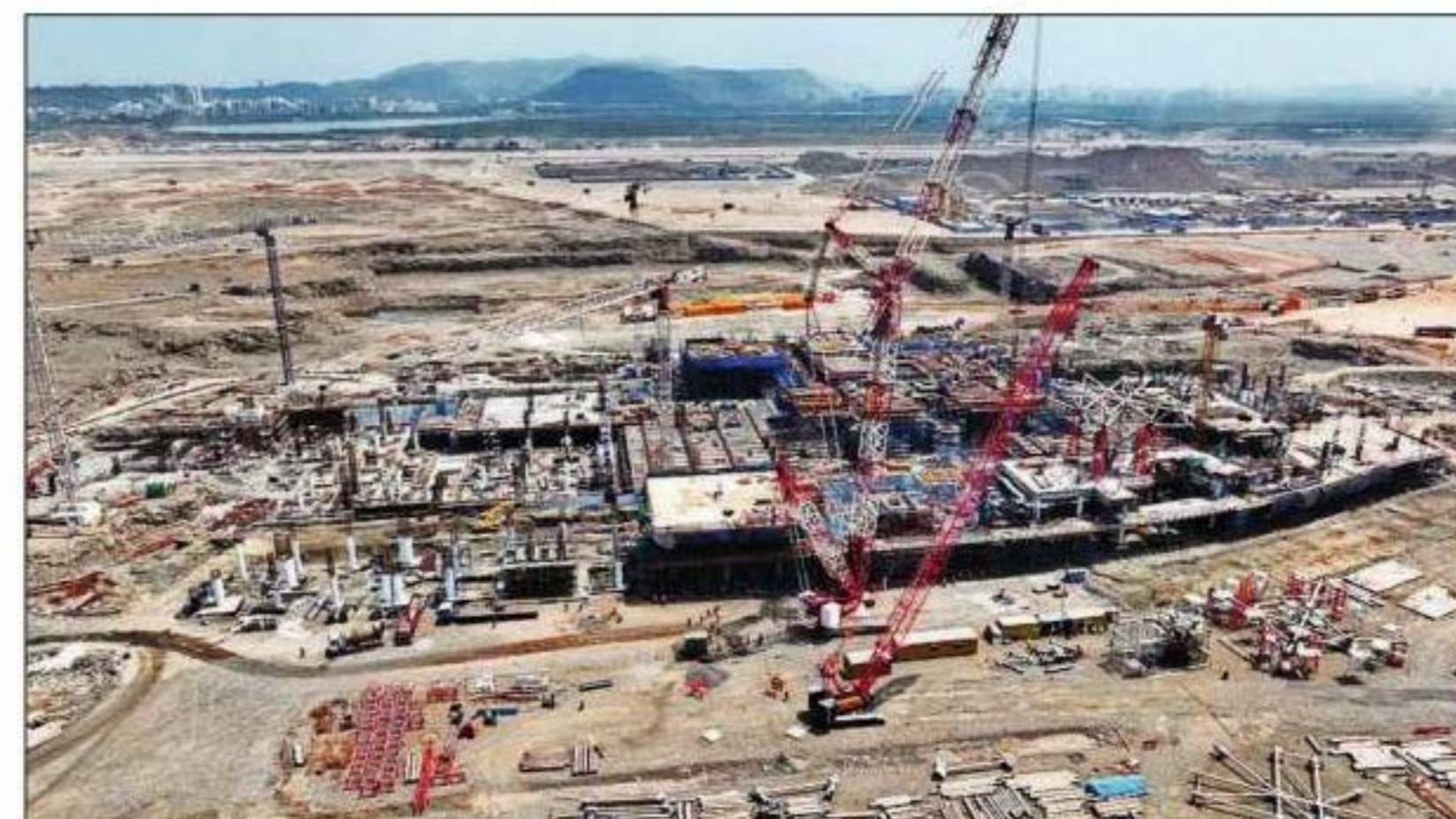
LEVIATHAN: NMIA is proposed to house India's largest general aviation terminal, with parking for 360 aircraft. At commissioning, parking for 60 jets will be available, straightaway easing the region's parking bay shortage woes
