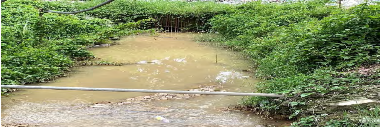
Storm water channels.
