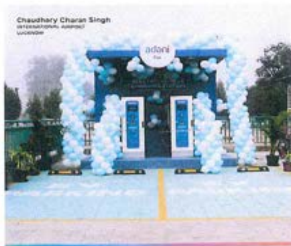
EV Charging Station
